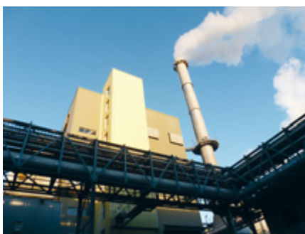
The biomass boiler produces green electricity. This is achieved through the use of biofuels which supply the boiler, and the purification of flue gas.
